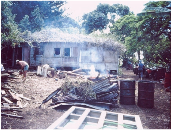
Fig. 8.1 A Pitcairn Island house being dismantled in April 1998 (Courtesy of Martin Gibbs)
